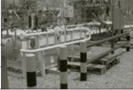
LEFT Orca Exploration continues to increase the capacity of its low-pressure gas distribution system by adding pressure reduction stations.
